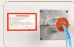
Installation of putty and application of identification label completes pass-through firestop. Putty holds cables in position, helping to prevent cable slippage and movement.
